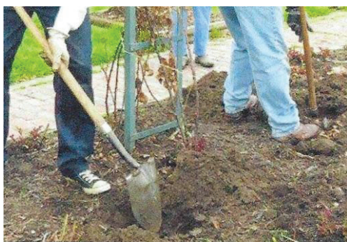
B-1 Dig hole eighteen to twenty (or more) inches deep and wide.
